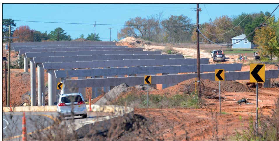
Work crews with the Texas Department of Transportation have been busy during the past several weeks working on Farm-to-Market 16 west of Lindale. The project covers an area four miles west of FM 849 east on FM 16 to downtown Lindale. Crews have been preparing the right-of-way by removing trees and grading embankment. The contractor is Highway 19 Construction, LLC and work is expected to be completed by the summer of 2025 at a cost of $4.4 million. Other work on the roadway includes grading, asphalt base, asphalt surface overlay paving, storm drain, bridge, and culvert structures, signing, pavement markings, and signals. Photo by Terry Cannon
