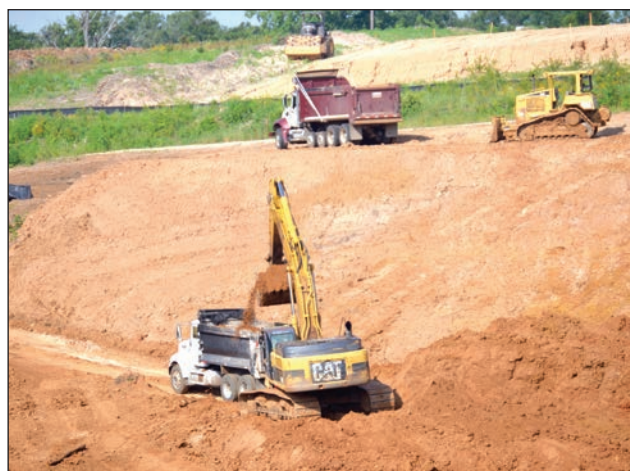
Dirt continues to be moved along Highway 16 west of Lindale as Texas Department of Transportation crews continue work this week. (Photo by Terry Cannon)
